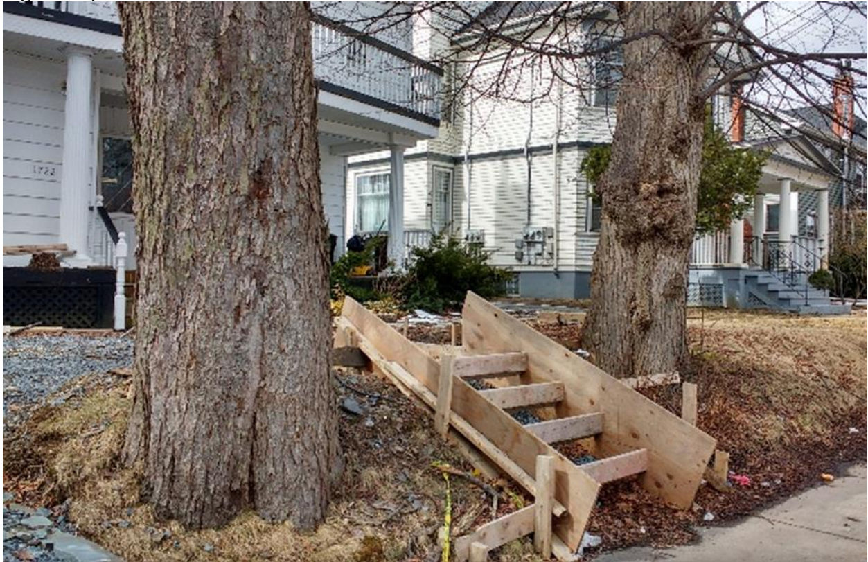
Photo 1a. Infrastructure installation beside Robie St. in Halifax. A new staircase plus driveway paving. Photo by James Steenberg, date unknown.
